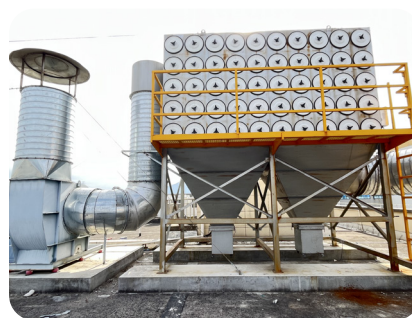
Welding Exhaust Gas Treatment Facilities (Newly-added)
