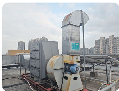
Fume Treatment System (Original)
